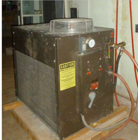
Figure 22. Picture of the Schreiber 300-AC 10.6 kW recirculating water chiller located in the basement of Building 470. Equipment courtesy of the DTRA TEAMS site at KAFB, NM.
